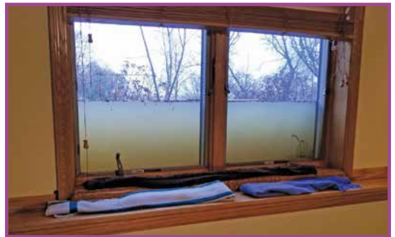
▲ In a job Petrasek will never forget, he responded to a home being inundated by floodwaters. Water was ponding halfway up the windows of this room, but Petrasek told the customer no amount of pumping would help the situation. (Photos courtesy of Lance Petrasek)
