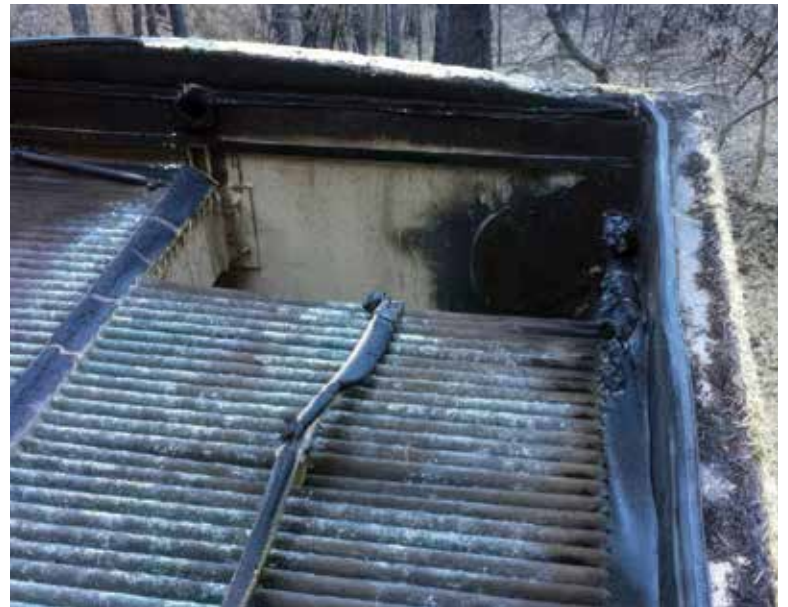
▲ The wildfire damage is extensive to an aboveground Orenco Systems AdvenTex AX treatment system.
