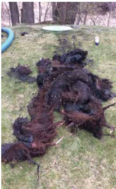
This huge clod of tree roots was pulled out of a malfunctioning septic system.
