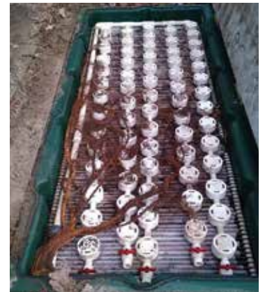
▶ Roots intruded on this AdvanTex treatment unit and will cause treatment problems if not removed and future root intrusion prevented.
