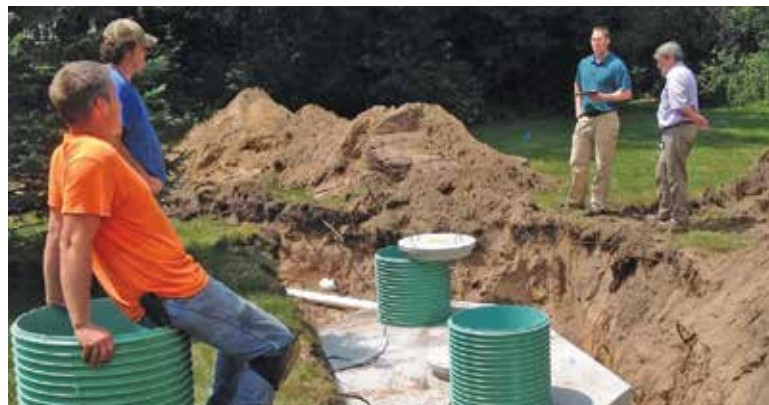
▲ Jake and Chris Bell and county inspectors Pete Ganzel and Alex Pepin looking at a pressurized mound installation. Risers are from Orenco Systems, tanks and lids from Wieser Concrete Products.
