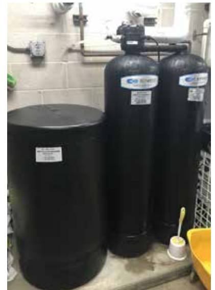
▲ This is a twin-tank system, one type of water softener that should be considered for use in a property utilizing a septic tank.
