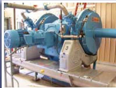
Fournier Rotary Press Dewatering
