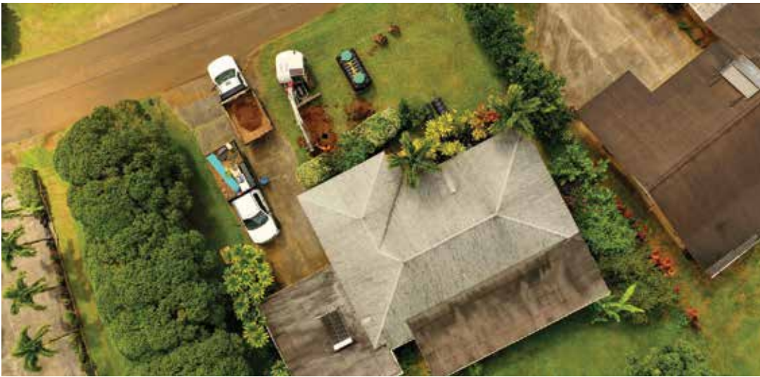
▲ An aerial view shows the small project site in Kapa'a, Hawaii, as work begins. A small septic system and mulch basin were both fitted into the front yard. Component outlines are visible on the grass.
