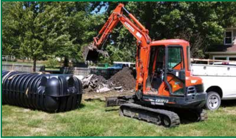
▲ A Roth North America plastic septic tank is installed with a Kubota KX121-3 mini excavator.
