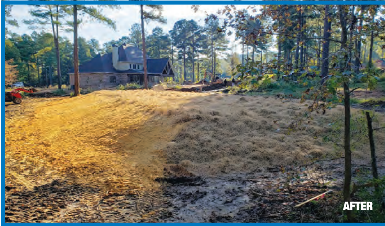
⬆ Before and after — the challenging installation of an ADS Septic Stack mound system, a bundled pipe product.
