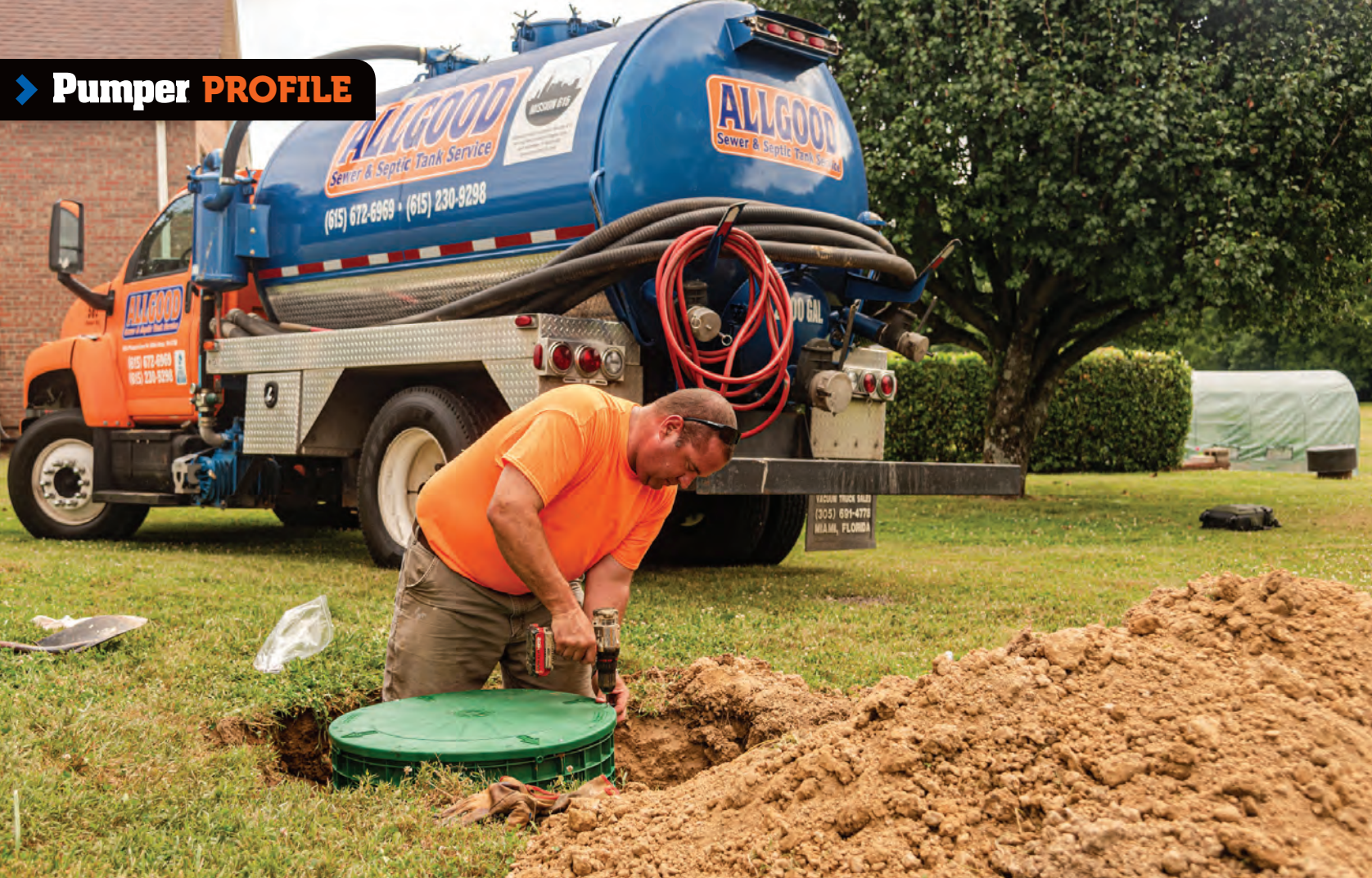
▶ Burge completes a Tuf-Tite lid and riser installation, bringing septic tank access to the surface for easier maintenance in the future.
