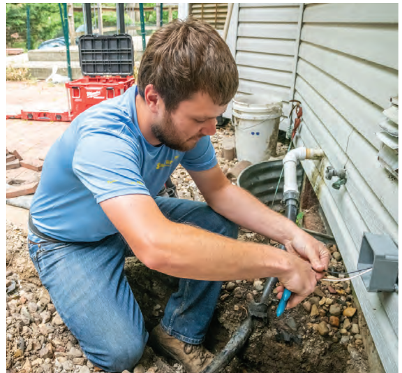
Dylan Link connects electricity to run a blower in a new system.
