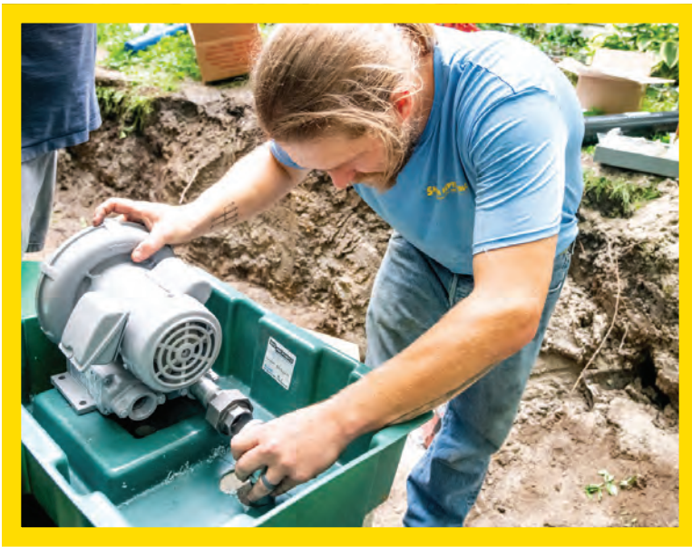
Colin Smith installs a blower from BioMicrobics for a residential septic system.
