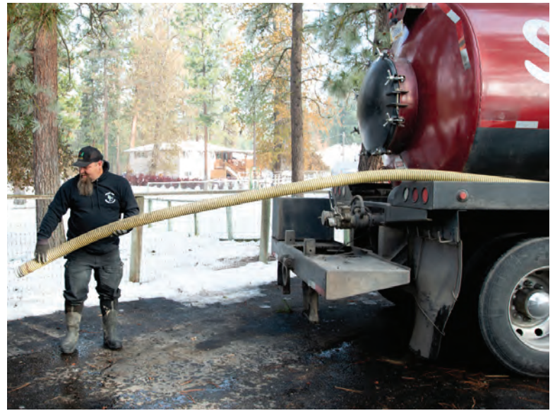
Service technician Nate Burkleo pulls suction hose from his Kenworth truck in preparation for a residential septic service.
