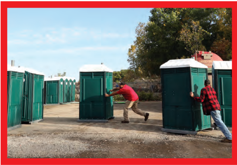
Charles Cross, left, and John Fowler arrange new restrooms from Satellite Industries in the company yard.
