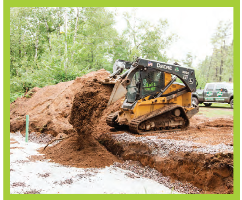
Below: Devin Lafond is at the controls of a John Deere tracked skid-steer during a septic system installation.
