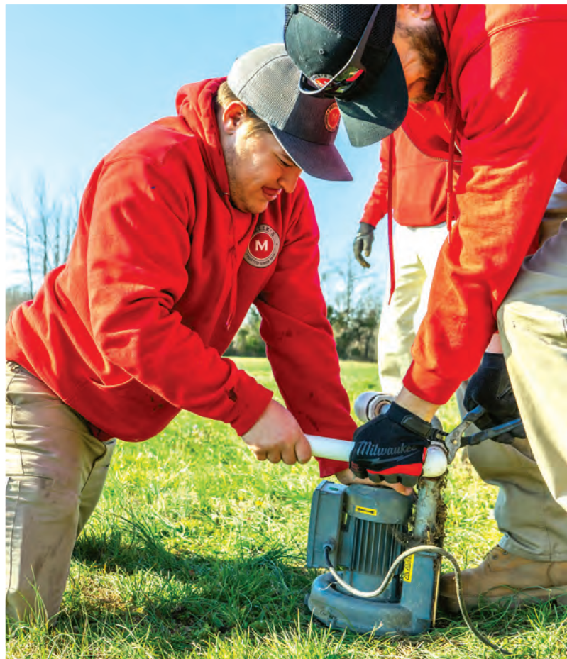
Technician Pierce Rained replaces PVC piping to an air pump before replacing it in the tank. At right, Kenney Boyette helps out.
