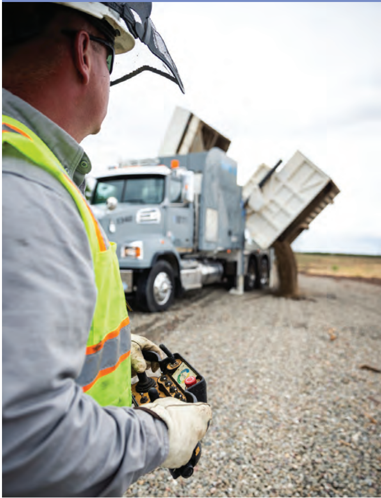
Left: Shawn Addison looks on as he uses the truck's remote to dump the debris from the box of the truck. One of the key features of the Dino is its ability to side-dump spoils.
