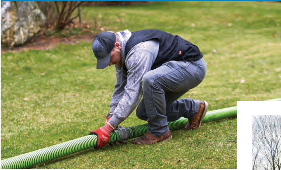
Left: Jeremy Giard connects suction hoses to reach a customer's backyard tank.
