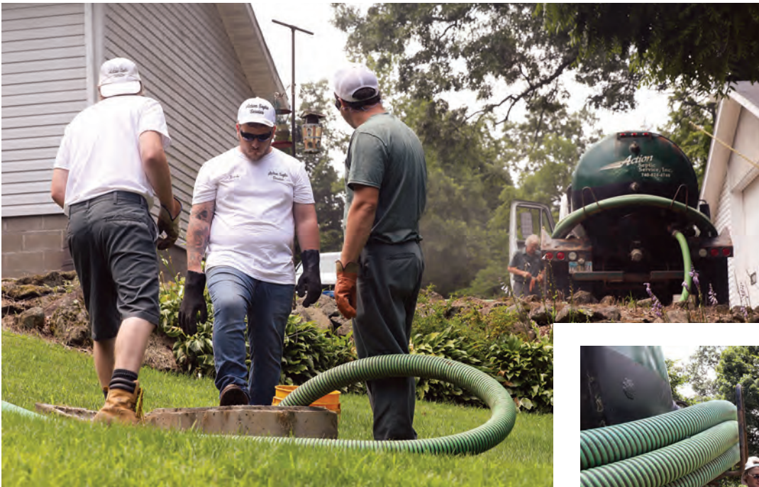
Left: The crew is at work pumping a residential septic tank. Malcolm Kettler (left), Zack Williamson and Evan Ehman manage the suction hose while Tim Kettler is at the truck.
