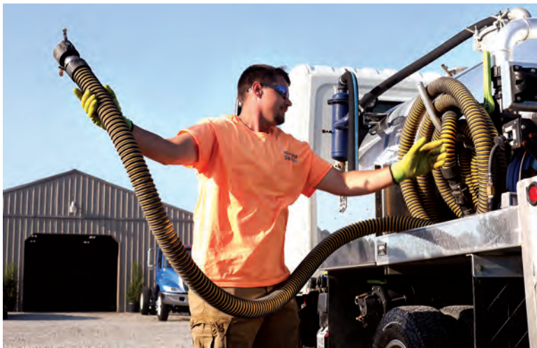
Technician Beau Nystrom prepares to service a restroom at a commercial work site using a Hino truck with Bruder tank and National Vacuum Equipment pump.
