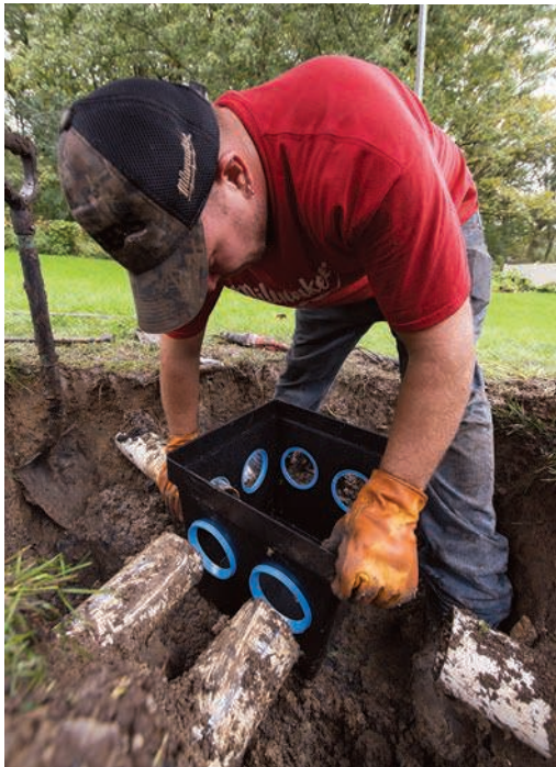
Left: Chris Haniford, a member of the septic/sewer crew at Feikema Plumbing & Sanitation, replaces a crumbling concrete distribution box with a TUF-TITE unit at a residential site.
