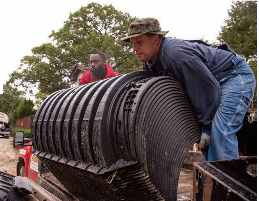
Below: Darrell Smith, left, and Kyle Arnold unload Infiltrator Water Technologies chambers for an installation project.
