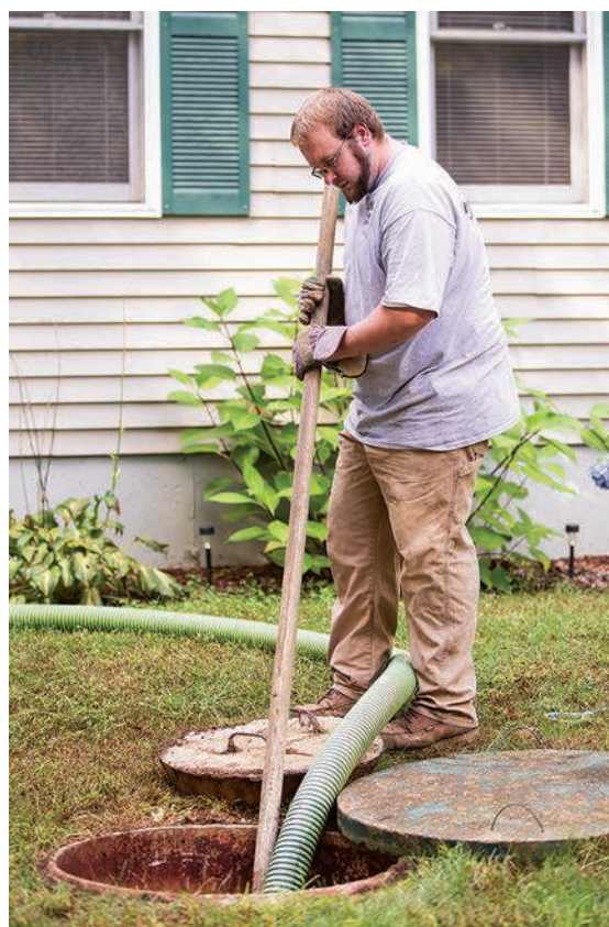
Below: Wyatt Alm agitates the contents of a septic tank during a pumpout.
