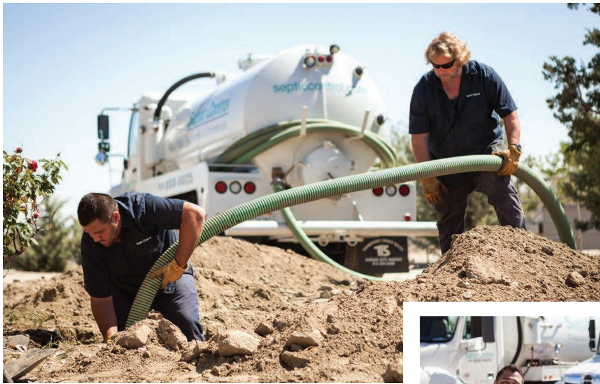
Left: Tony Diaz, left, and Wayne Higgins pump a septic tank using a vacuum truck from Transport Truck Sales and using a Masport pump.
