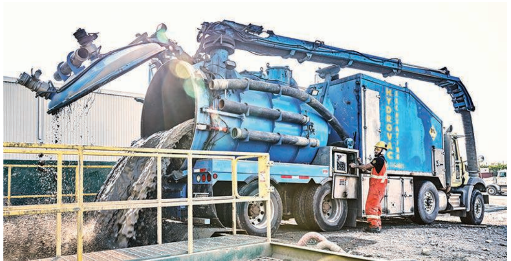
A technician for Ontario Excavac dumps a load from a hydroexcavation truck manufactured by Transway Systems.
