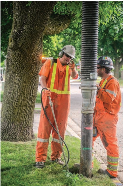
Technician Scott Langdon pauses to give instructions to Justin Levert as the pair operate a Vacall AllExcavate hydroexcavator with a Roots blower from Howden.
