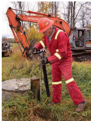
Shaw removes improperly installed electrical conduit in preparation for a tank replacement. His Hitachi Zaxis excavator is shown in the background.
