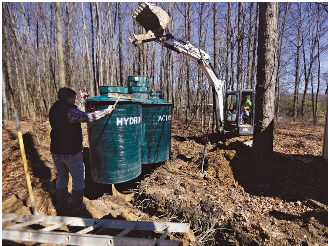
Left: Operator Marty Pero uses a Bobcat E55 compact excavator to lower a Hydro-Action unit into the ground during a system build. Also shown is James Dye, owner of Wastewater Solutions, a Hydro-Action distributor.
