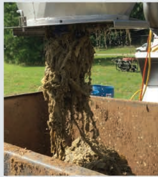
BEAST screening discharge from Vector Truck.
