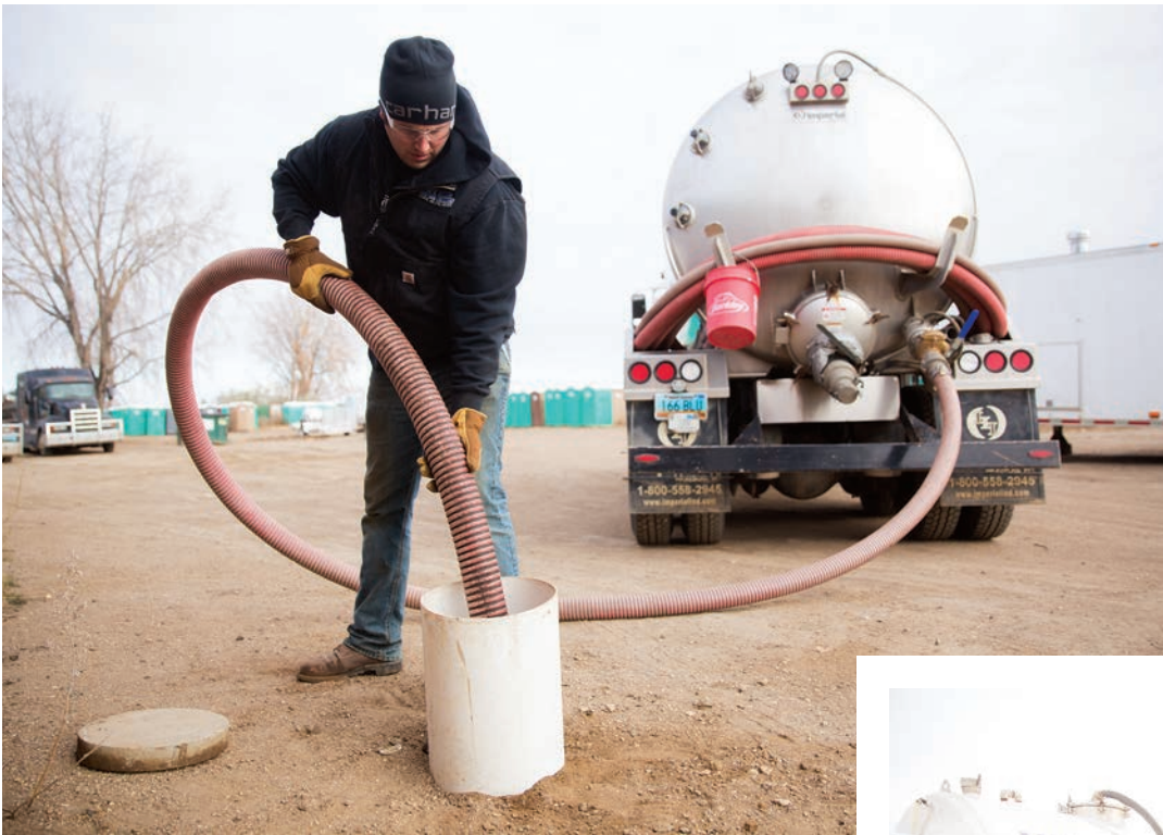
Left: Reid Hanson pumps a residential septic tank near Minot, North Dakota, using a truck outfitted by Imperial Industries and running a Masport pump.
