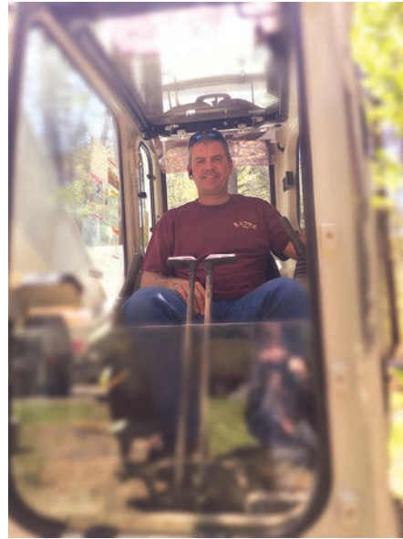
Above: The R.M. Ratta crew is hard at work installing driplines at a residential property. They are using a Link-Belt 225 excavator to complete the project.
