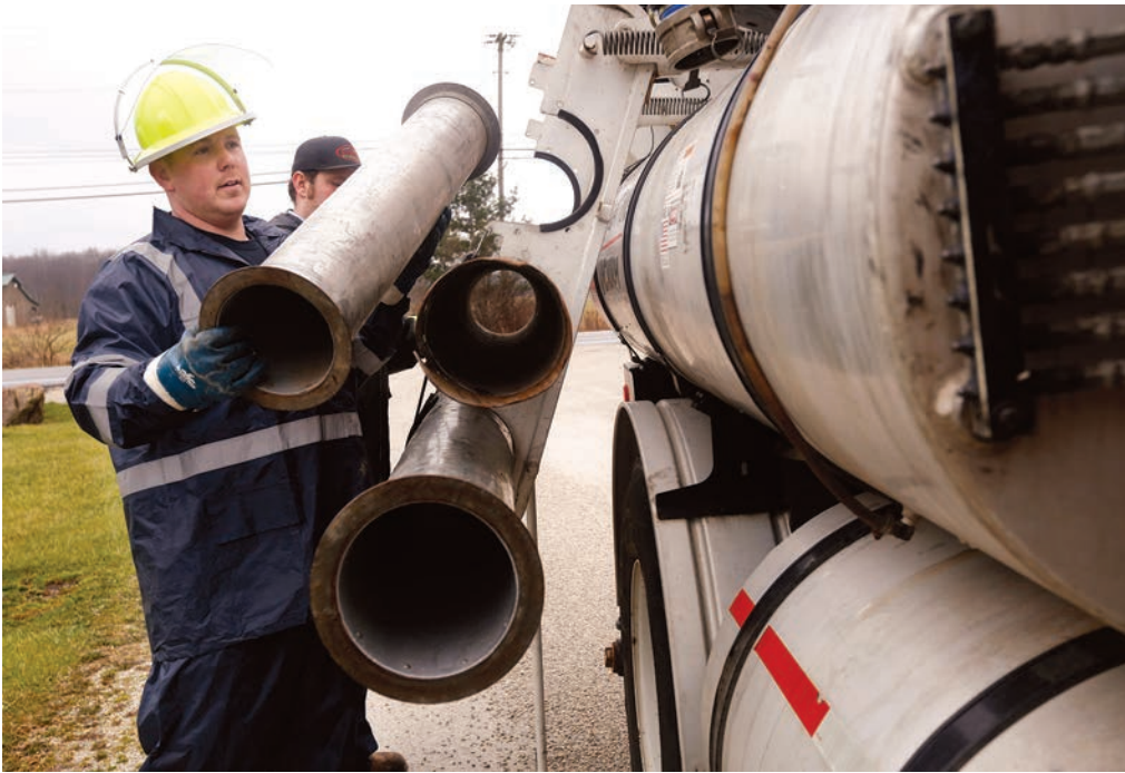
Left: Kyle Dye, left, and Rex King Jr. get ready to assemble the boom on a Vactor 2110 combination truck.
