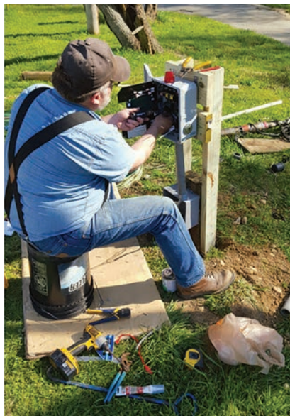
Eddie Harrison rewires control panel.
