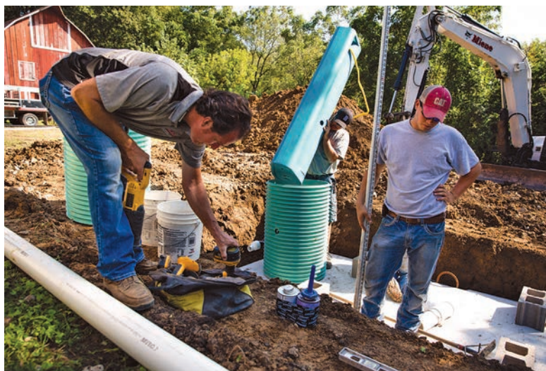
Above: Rick Miene, Anthony Schmitz and Dylan Jacobs install components of an Orenco AdvanTex system at a home in Cedar Rapids, Iowa.
