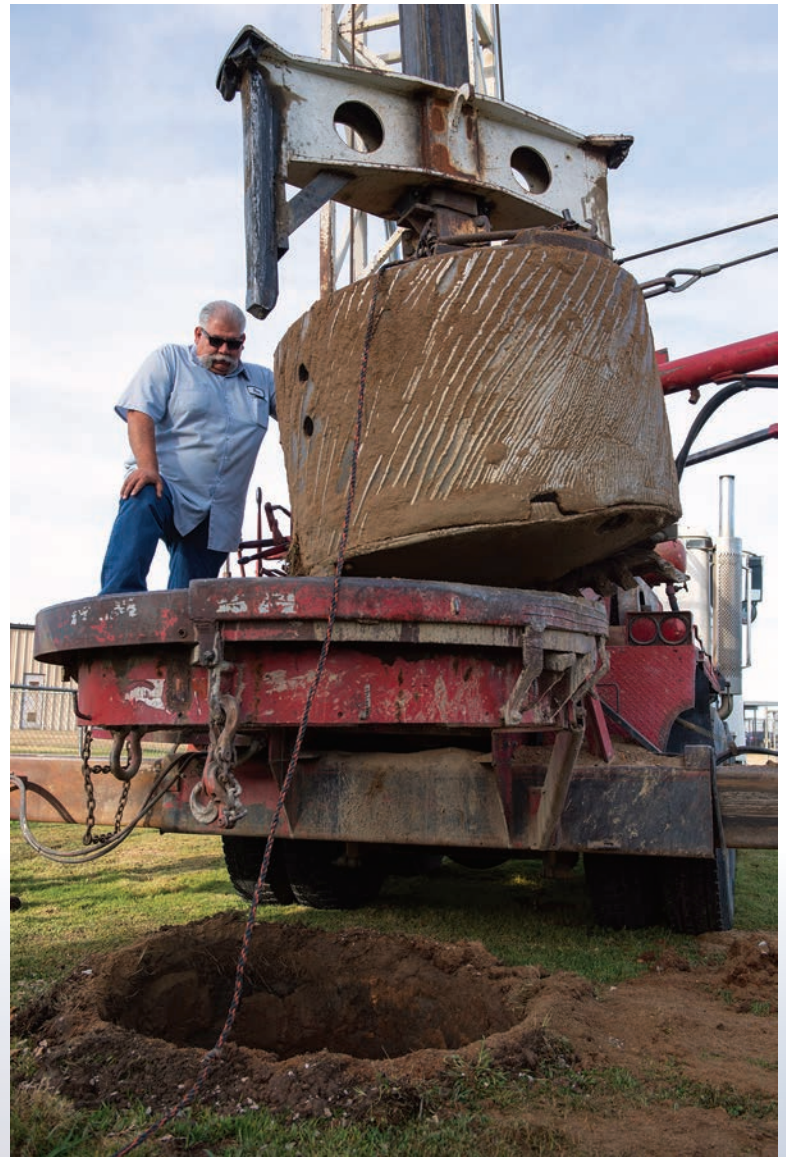
Above: Foreman Marcello Ruiz checks the Calweld drill rig on a job site.
