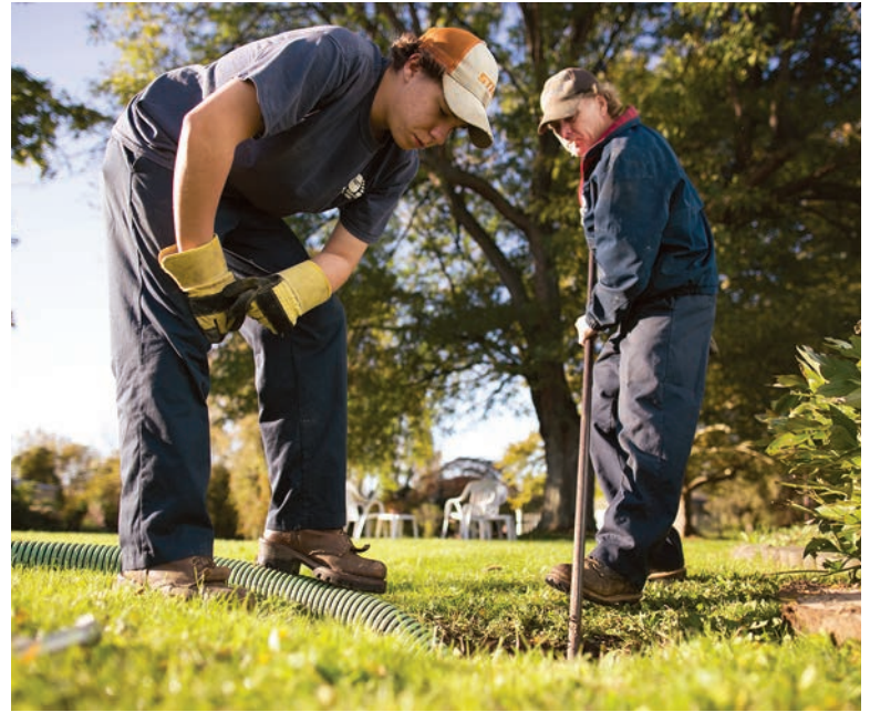
Below: Technicians Cole Johnson, left, and Kevin Walton empty a septic tank in Scottsville, New York.
