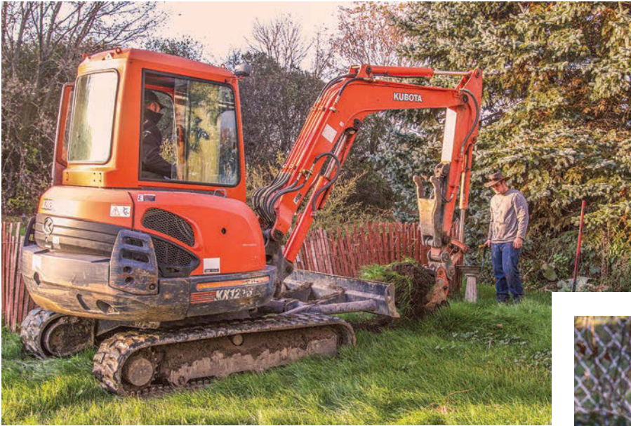
Left: Mike Clark works in a new trench while Billy Clark helps in the background.
