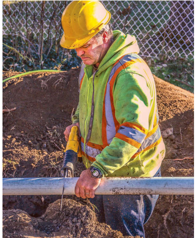
Below: Mike Clark cuts PVC pipe during a septic system replacement in Bethany, Ontario, Canada.
