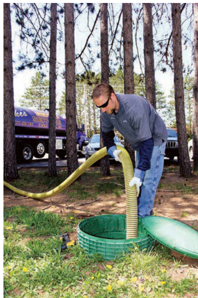
Steve Nobble prepares to pump a commercial holding tank. The lid and riser are from Tuf-Tite.
