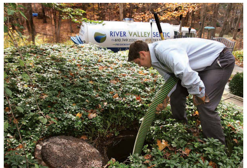
This tank is well-camouflaged, surrounded by landscaping. Wilson dragged his hoses up a walkway to reach the tank in Ottsville, Pennsylvania.
