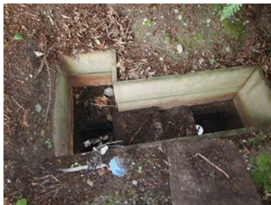
During a follow-up inspection, Alan Chapin found an interior electrical box used outdoors and no cover over a makeshift wooden frame exposing tank access lids. (Photos courtesy of Alan Chapin)
