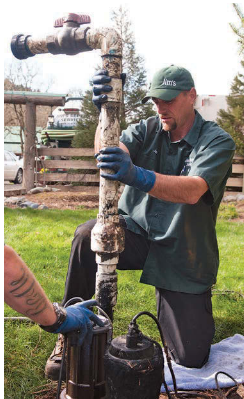
Left: Joshua Fiske replaces a failed pump with a 280 Series Liberty pump during a septic service stop at an Oregon home.
