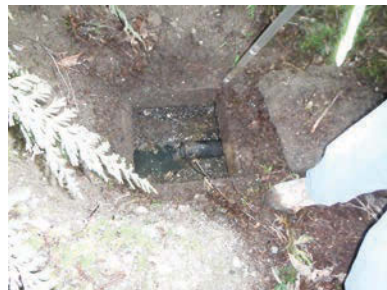
According to Alan Chapin, this tank received an OK from a previous point-of-sale inspection. The inlet baffle was missing and an inadequate 3-inch ABS pipe was used.
