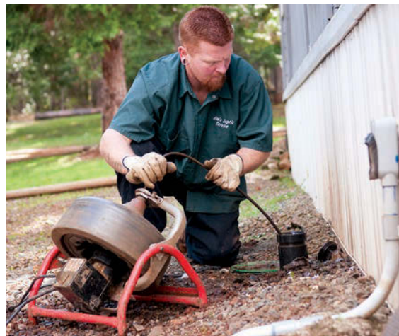
Below: Technician Doug Modgling uses a RIDGID K-3800 Drum Machine to snake through a clogged line running to a septic tank.
