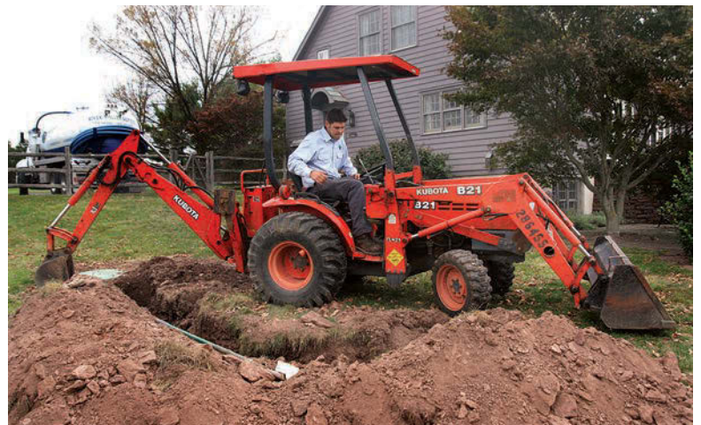
Wilson uses his compact Kubota backhoe loader to excavate a pipe during a repair call.
