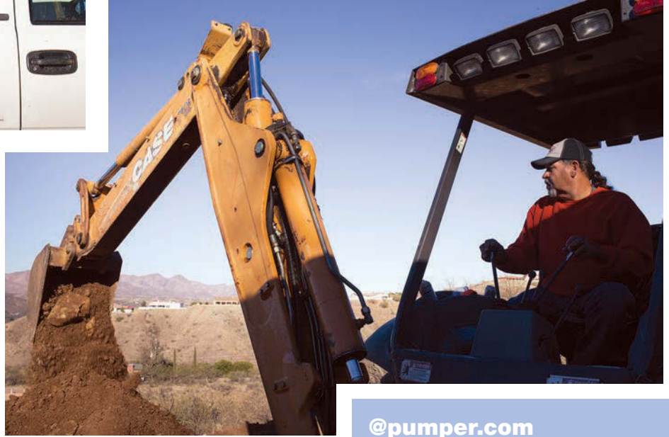
Below: Ruben de la Rosa II operates a Case backhoe during a septic system installation.
