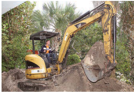
Reliable machine operator Seth Record uses a Caterpillar excavator during a drainfield installation.
