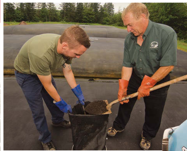
Francis Overmars, right, and his son, Mark, inspect solids during dewatering. The company uses geotextile dewatering tubes supplied in Canada by Syn-Tex and Terratube for the job. The tubes are 45 feet in diameter and 80 feet long.
