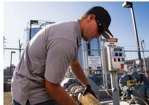
Technician Lance Brown hooks up his hose to off-load a load of grease trap waste at a FOG disposal site at the Sacramento Regional County Sanitation District.
