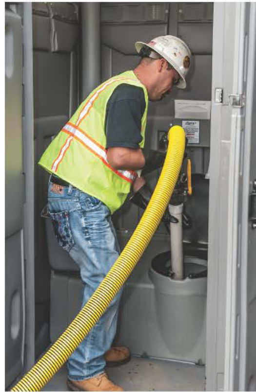
Juan Perez pumps the holding tank of a restroom in the company yard. Technicians including Perez evaluate each other's performance to ensure quality service.
