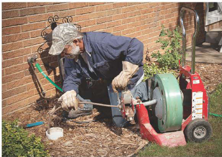
Joseph Threm is rodding out the sewer line from the house to the tank with a Spartan Model 300 cable machine.
