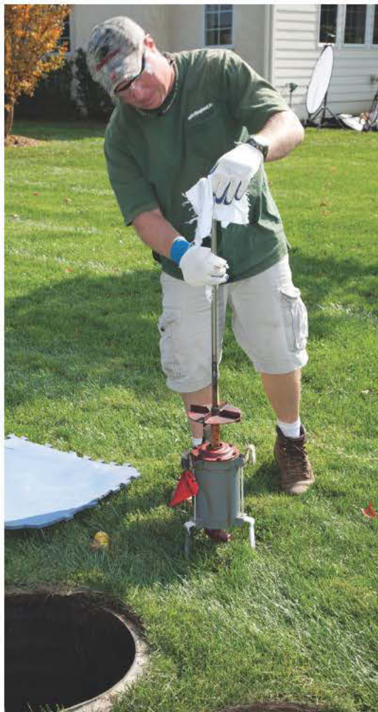
Field services technician Dave Burgess checks and cleans an aerator motor from Jet Inc.
