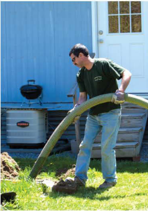
After hand-digging this 500-gallon residential septic system, Sean O'Brien gets to work pumping.
