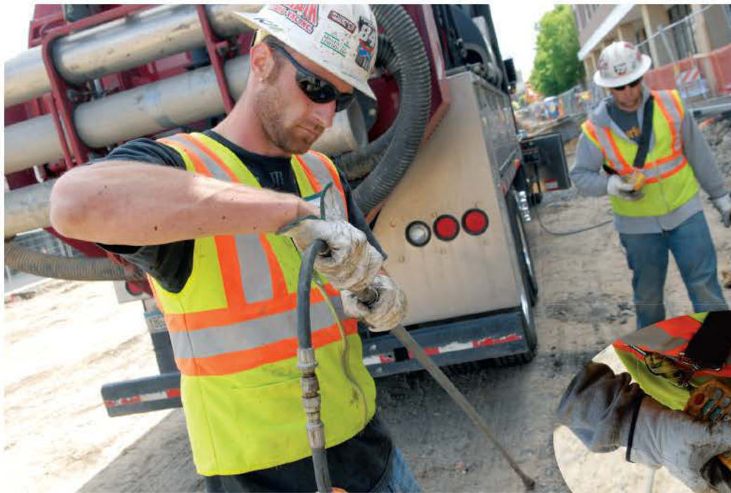
Mike Doerfler (foreground) and Jeremy Doerfler put away tools after finishing a job at the site of the light rail line in Minneapolis. (Right) This wireless remote controls the vacuum and jetting capabilities of the Vactor truck. Brandt Volk says the remote is a valuable accessory upgrade for his crews. (Photos by Stephen Gefre)
