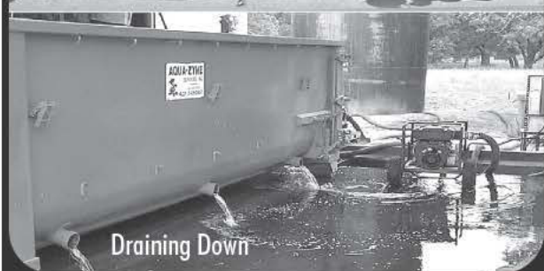
Filter Box Interior
