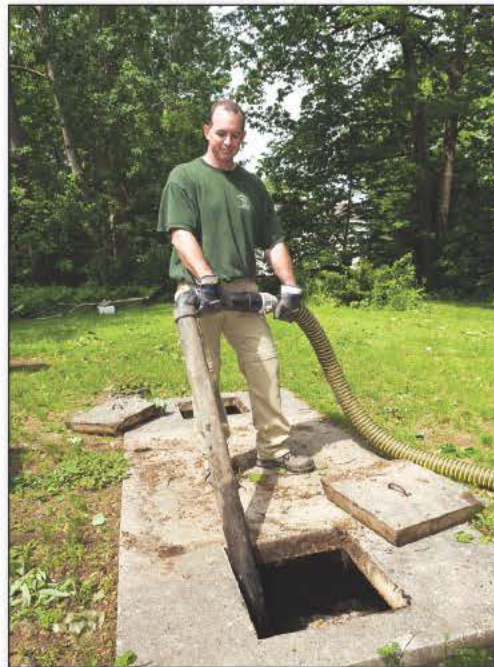
Keith Robillard uses a custom-made wand for pumping a dual-compartment tank. The wand is made from a 3-inch PVC pipe about eight feet long with a 90-degree elbow to allow cleaning tank corners better. A cam fitting attaches the wand to a Tiger Tail hose.
