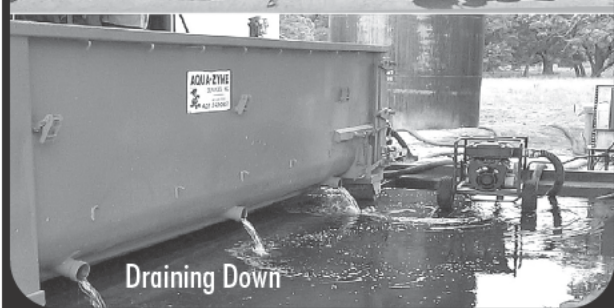
Filter Box Interior
