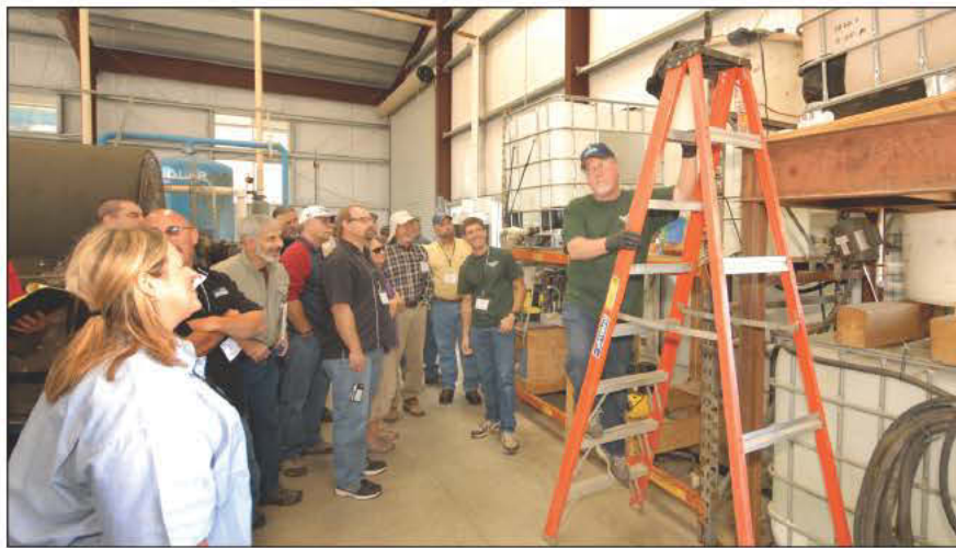
Plant manager Bob Hess prepares to mix filtered septage at a 10-1 ratio with polymer solution.
