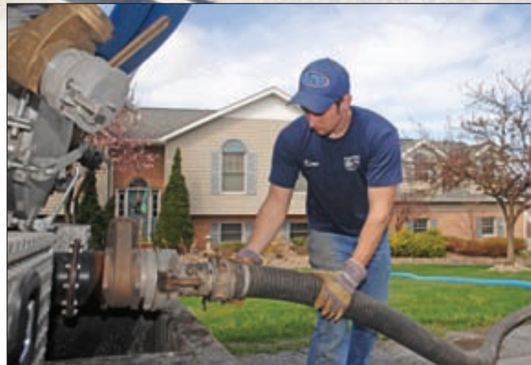
Wertz III removes a vacuum hose to his service vehicle after pumping out a residential septic tank. His crew pumps 10-12 tanks on a busy day.
