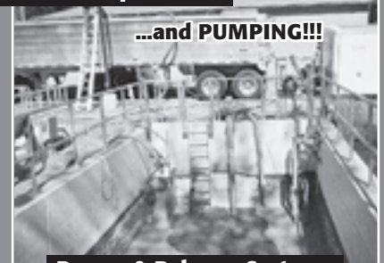
Pumps & Polymer Systems
