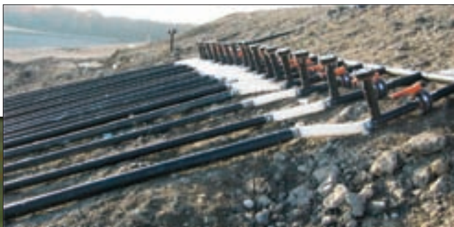
Four-inch perforated pipes are installed in the refuse mass to distribute septage liquid and speed up decomposition of the garbage.
