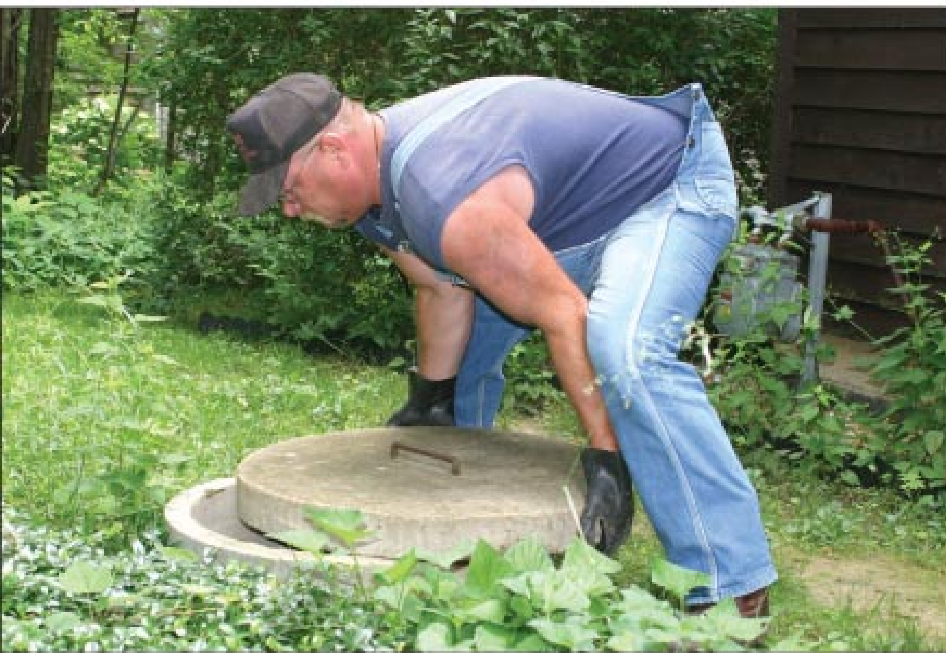
Bob Bond replaces a concrete lid on a septic system. Barnes Sewer & Septic believes the work doesn't stop when the tank is cleaned. They believe spending time educating customers is essential to providing good service.
