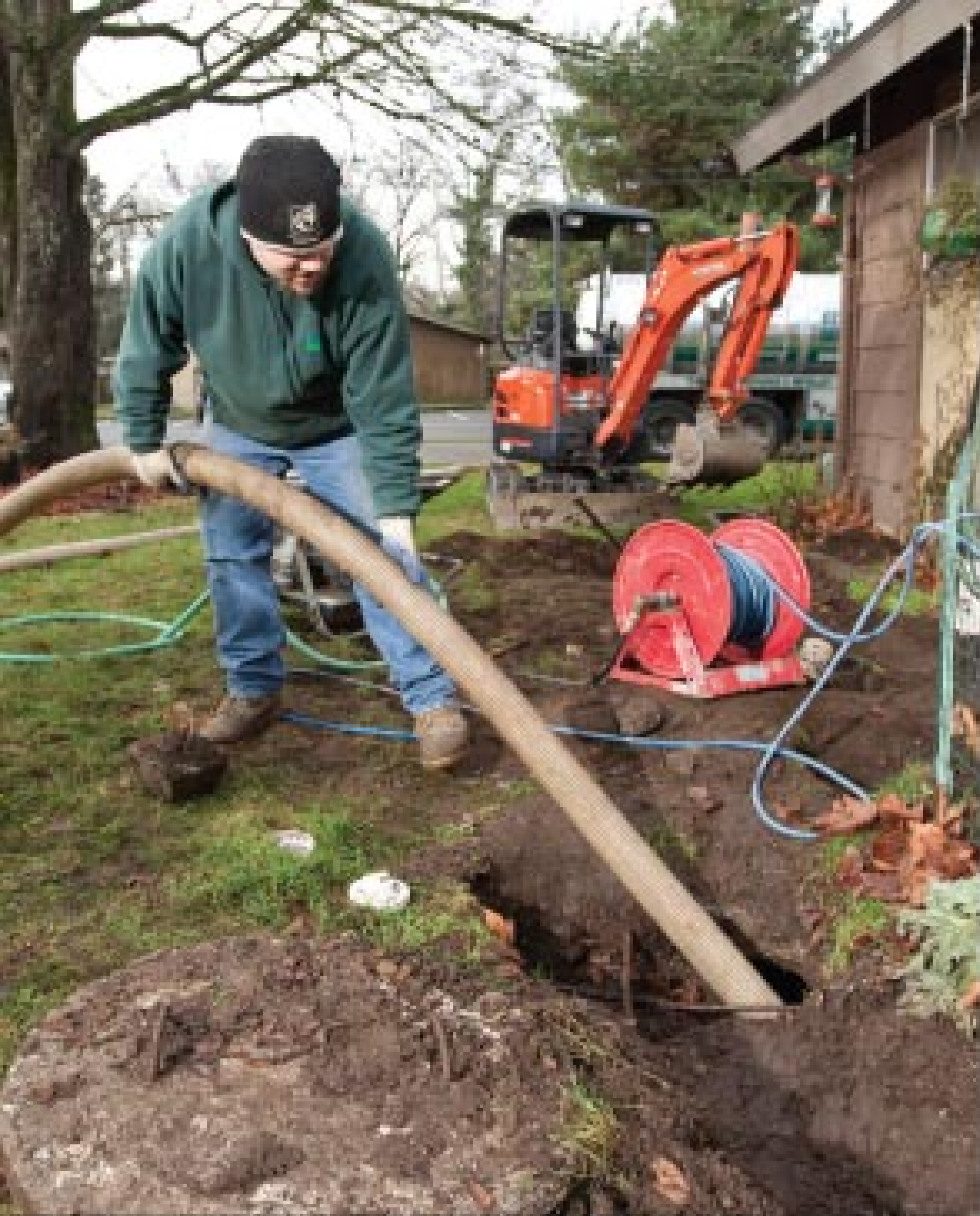
Long evacuates a septic tank so technicians can troubleshoot the cause of a failing septic system.
