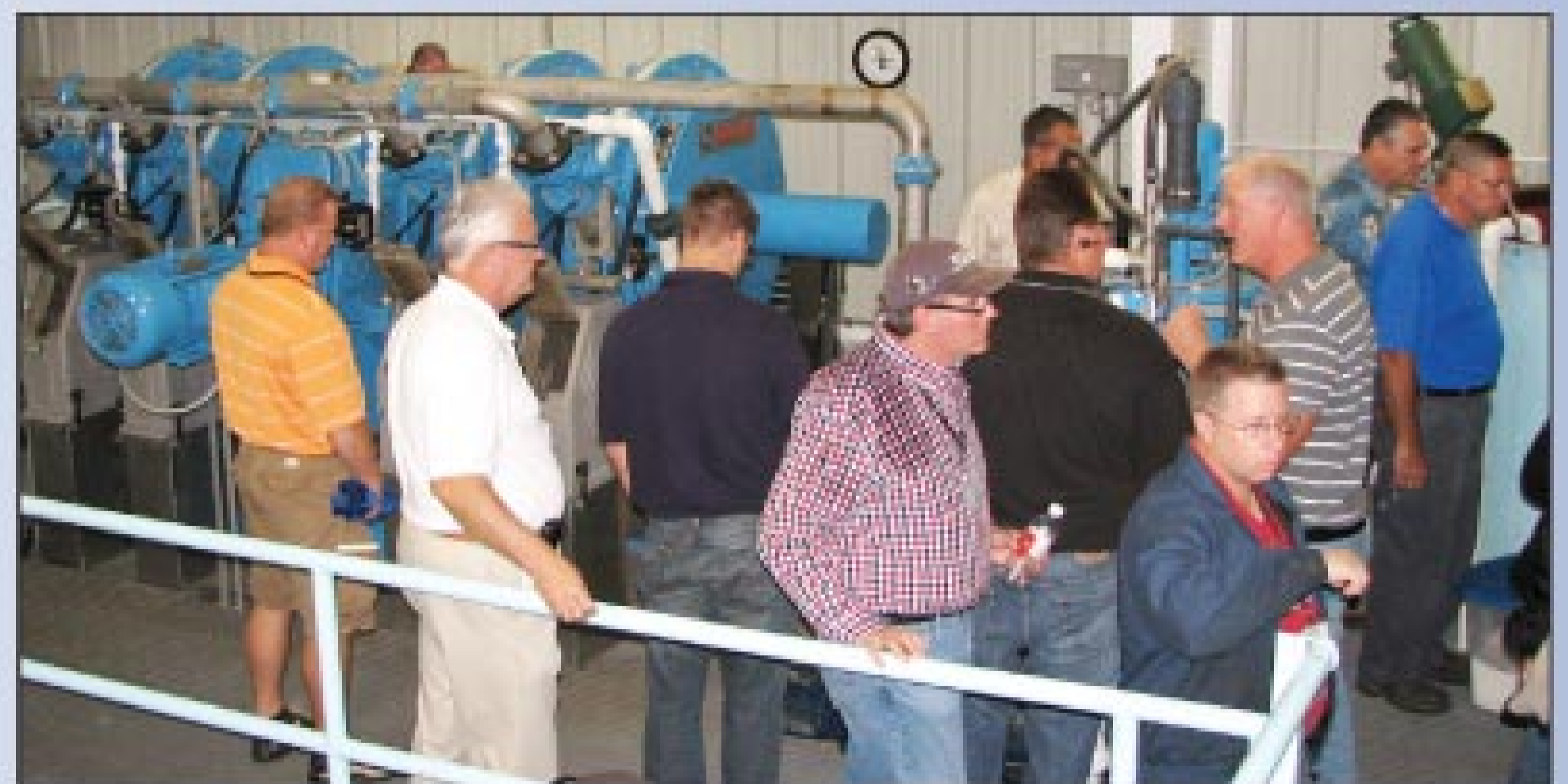
A Fournier Industries rotary press is a key component in waste processing at Hapchuk's Liquid Assets Disposal facility.
