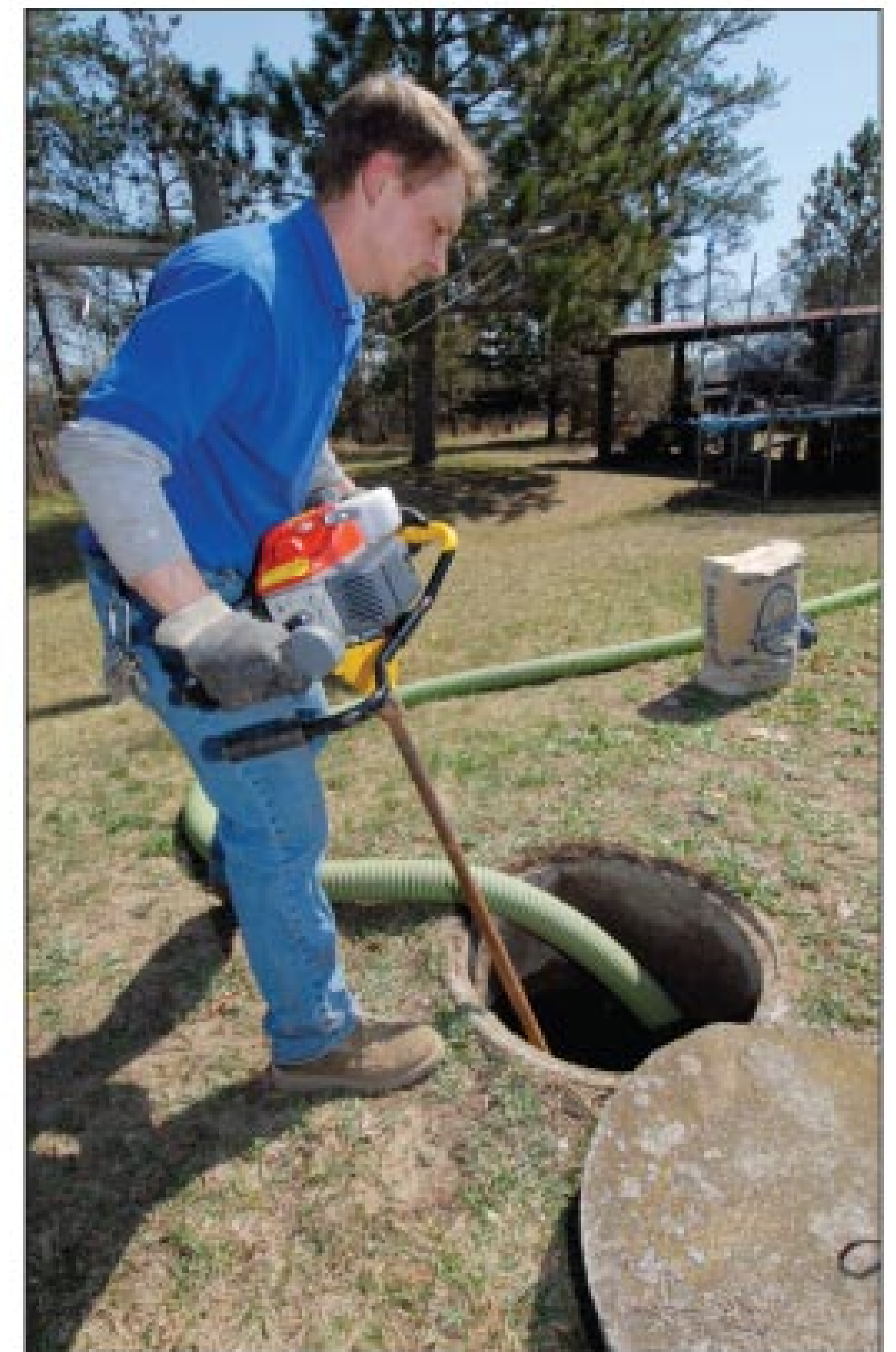
Johnson uses a Schmitz Brothers CrustBuster tank agitator to loosen septic sludge during pumping.
